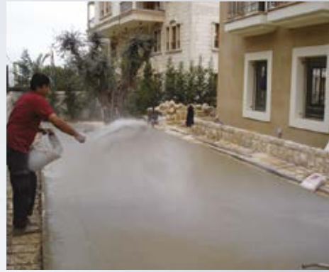
2- Dry Shake method to spread evenly the color Hardener on concrete wet surface
